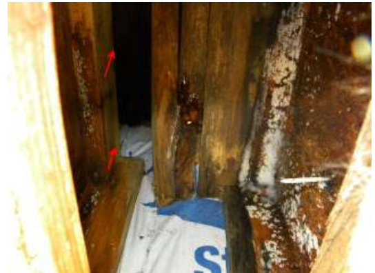
Water damage and mold under a deck
