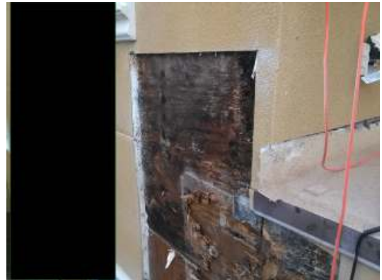
Rotted sheathing at a deck
