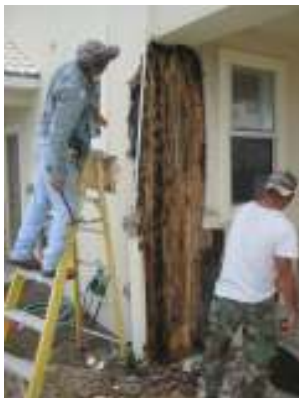
Wood sheathing rot behind hard coat stucco under a deck.
