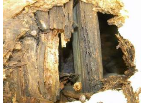
Wood rot under a deck
