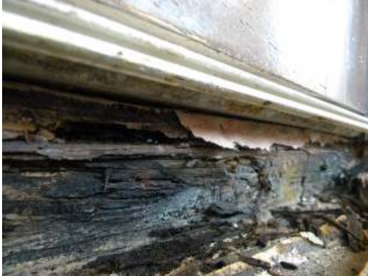
Wood rot under a deck door.
