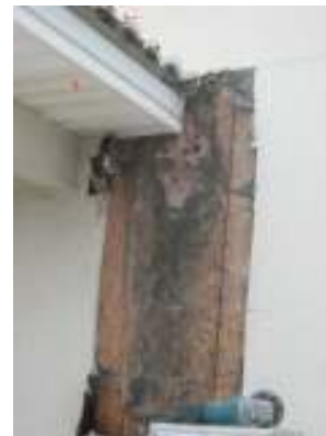
Wood rot from an improper kickout flashing.
