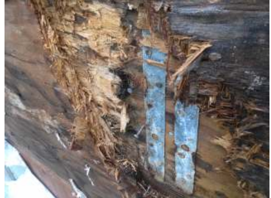
Rotted plywood under the stucco.
